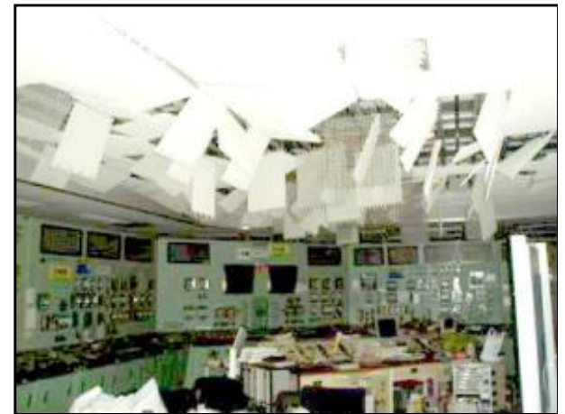
Unit 1 Main Control Room
